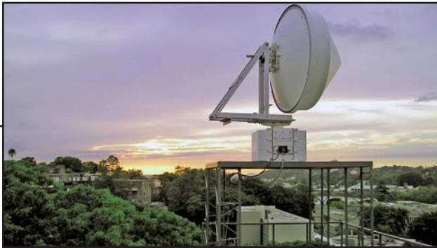
■ A CASA student-designed radar network being installed in Puerto Rico produces accurate rainfall data that will be used to predict flooding and support other applications such as crop hydrology that require accurate rainfall estimates.
