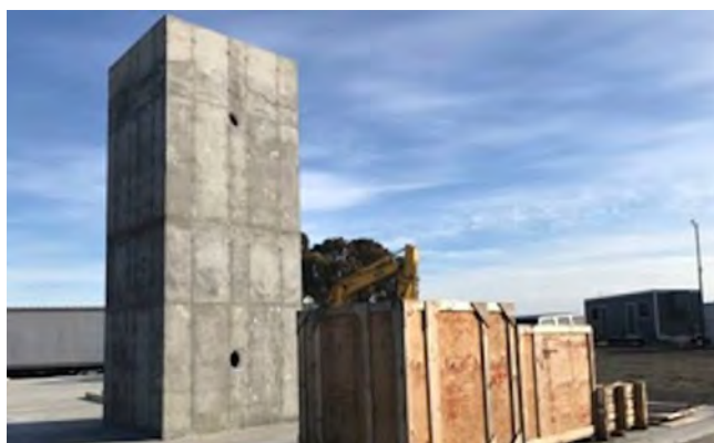
Figure 6-7: The bioreactor, shown here under construction at Silicon Valley Clean Water, will assess the benefits and performance of mainstream, full anaerobic treatment to facilitate energy savings and water reuse. (Credit: Eric Hanson, SVCW)
